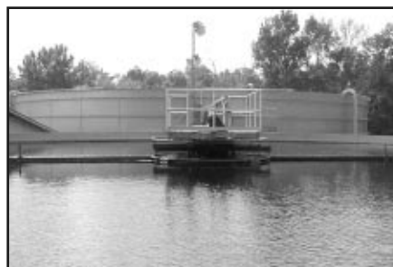
Figure 2. American Protein final clarifier.
